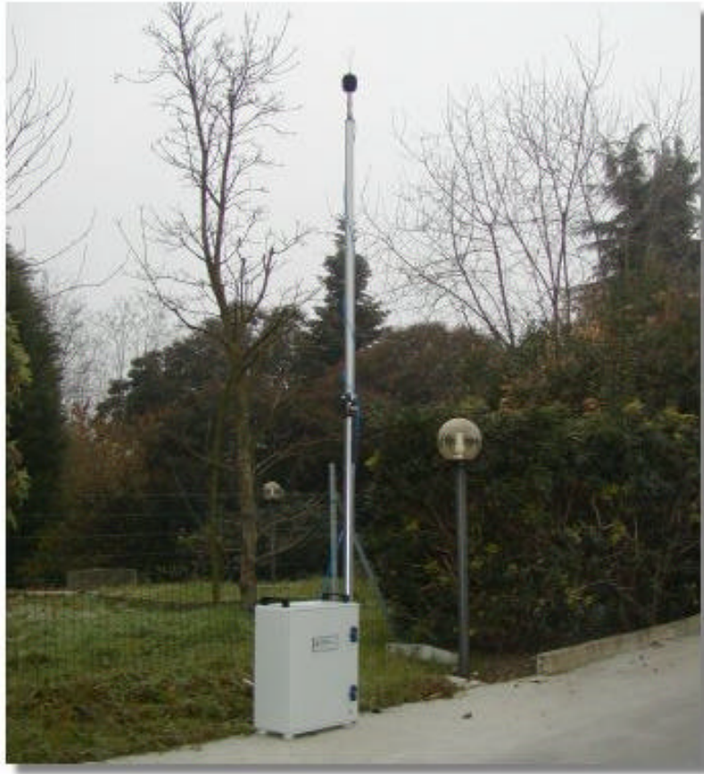
Figure 2 – Temporary battery operated installation with GPRS data transmission
