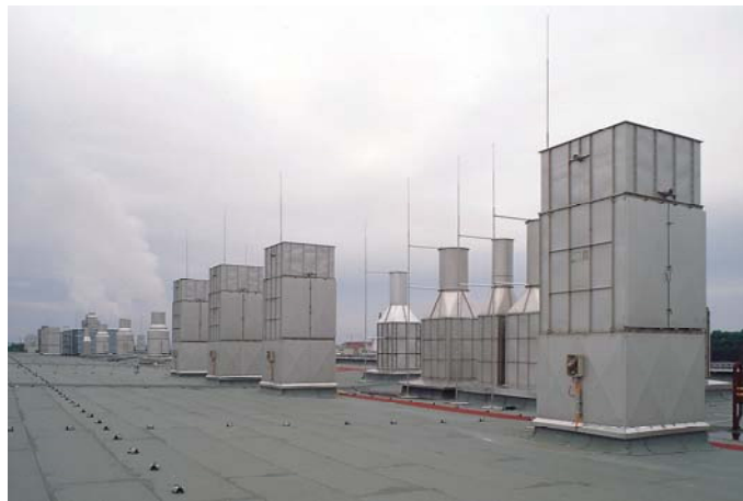
Figure 2 – Silencers on the building roof, Haindl Papier, Augsburg PM3
