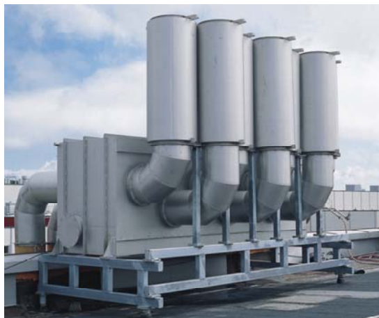
Figure 7 – Multi-pipe resonator and absorptive silencers for vacuum pumps
